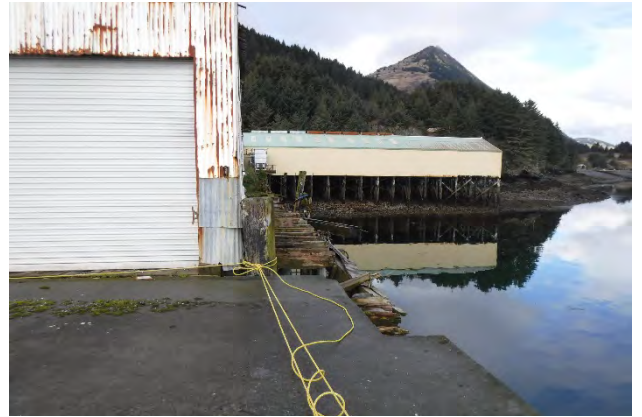
South view of missing/damaged dock
